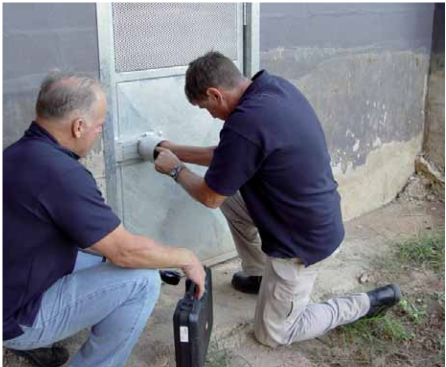
Greg Morrison and senior technician, Robert Guiffre, lock up access to the sub floor. The line along the wall clearly shows the level of soil, both inside and out, before they started clearing the premises of termites.
